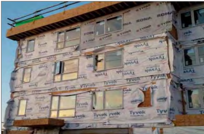
Figure 2.5 Poor House Wrap Installation
